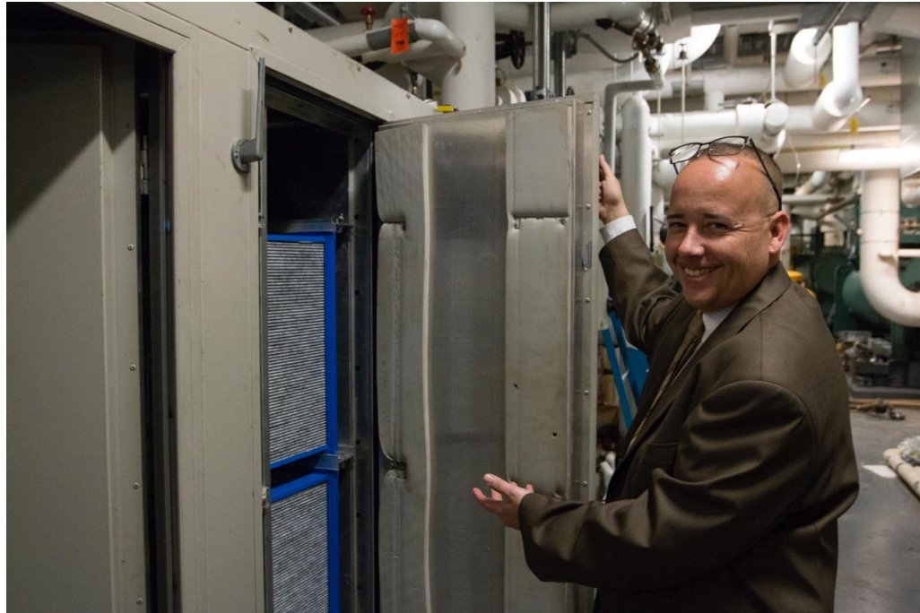
Nelson Nieves from building operations presents the air filtration system under the lobby floor. Image courtesy the Museum of Modern Art. Photo: Manuel Martagon.
