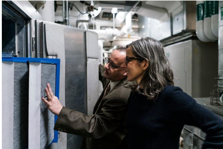
Ms. Katchadourian looking at the MoMA’s air filtration system with Nelson Nieves, assistant director of building operations. Credit An Rong Xu for The New York Times
